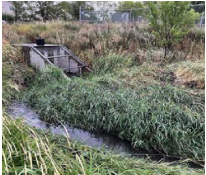
Figure 4. Outfall at KAL_AC6. Two pipes converge and discharge into the grassy channel. Picture taken August 8th, 2021.
